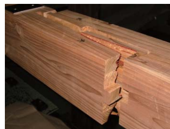
第8図 せん断破壊 Fig. 8. Shear failure of beam ( kanawa-tsugi joint).
