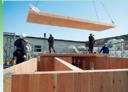
We have conducted various studies to put the new wood material CLT (cross laminated timber) made of Hokkaido timber to practical use and achieved CLT construction using domestic larch for the first time in Japan.
