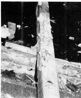
写真21 居間中央部に残された布基礎( )と土台( ) Photo.21. Hyphae and spores around the foundation ( ) and the sill ( ) left at the reconstruction .
