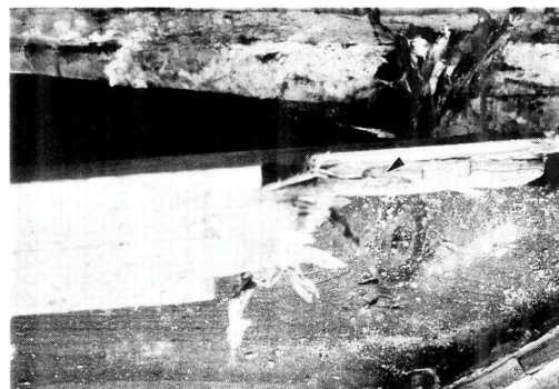
写真 16 CCA 土台の腐朽 ( ) 状態 Photo . 16 . A decayed wooden sill (CCA-treated) .
