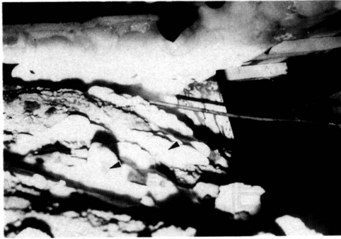
写真1 床下土壌面の菌糸生長(▶)と大引上の菌糸(○) Photo.1. Hyphal growth on the ground (▶) under the floor (○ hyphae on a sleeper) .
