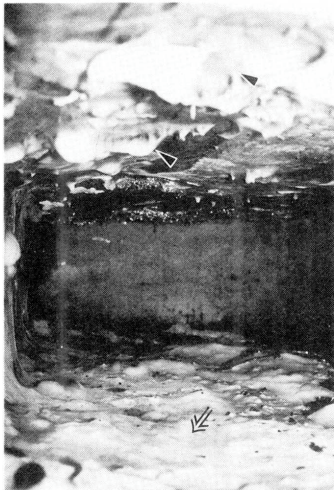
写真 6 床下熱断材受け (▶) と土壌面 ( ) の菌糸生長 Photo .6 . Hyphal growth on the ground ( ) and the supporting lumber (▶) for glass wool via a concrete foundation under the floor .
