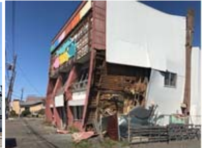
(c) 側面、壁の崩落
