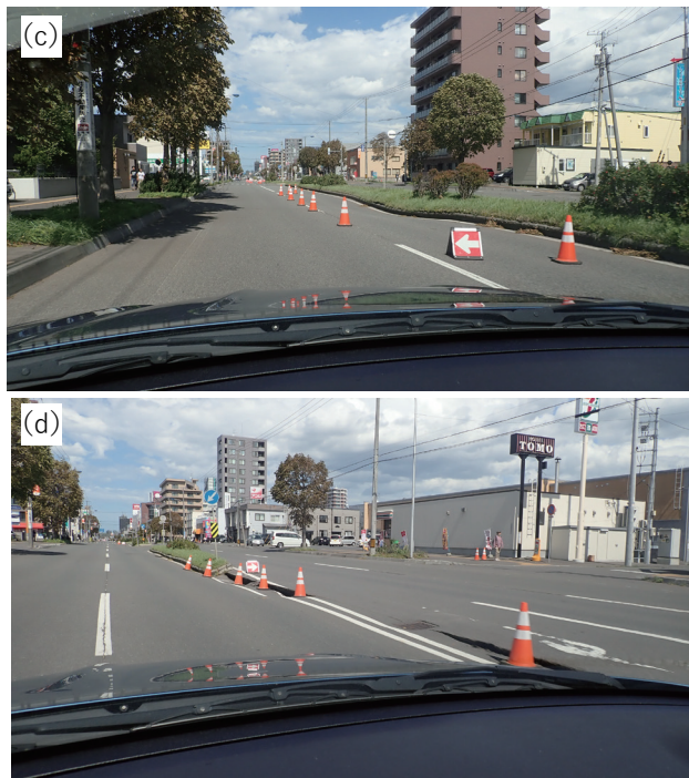
Fig. 10 Destruction situation of surface rupture between kita-29 jo and kita-44 jo, higashi-ku, Sapporo city.
