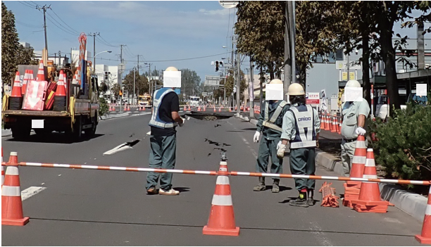
図12 東区北45条～北47条にかけての地盤変状状況 Fig. 12 Destruction situation of surface rupture between kita-45 jo and kita-47 jo, higashi-ku, Sapporo city.
